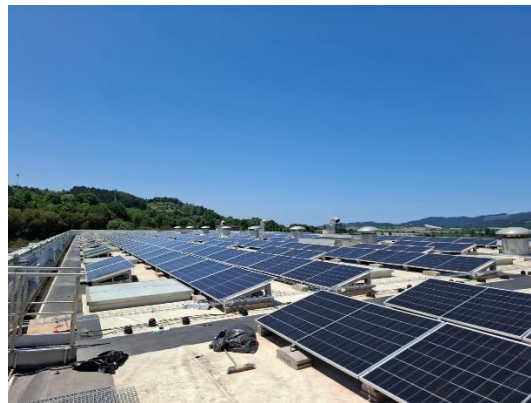
Figure 24. Photovoltaic panels of BATZ Zamudio installed in 2025
